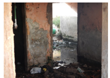
(Photo-3) An abandoned house in a flood prone area
