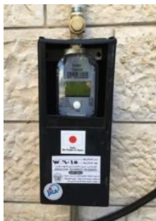
Figure 3: Photo of a Pre-Paid Water Meter
