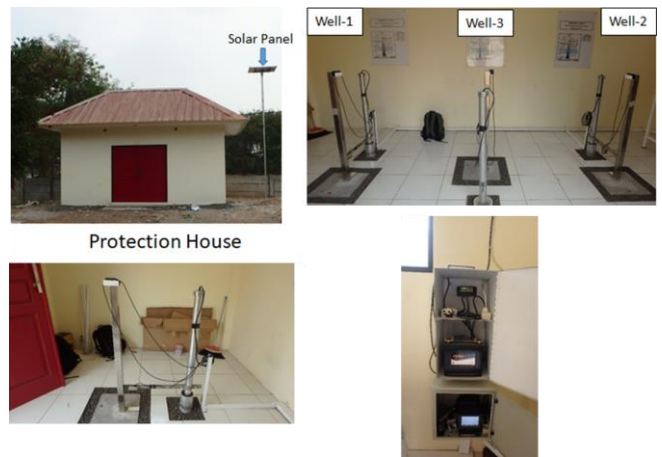
Figure 8 Land subsidence monitoring well
