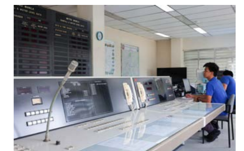
Rosario Master Control Station developed by the Nationwide Flood Control Dredging Project (Telemetering Portion). The volume of water in the river is properly controlled by judging the opening and closing of the Rosario Weir, and the beginning of the release of water is also warned about in the area.
