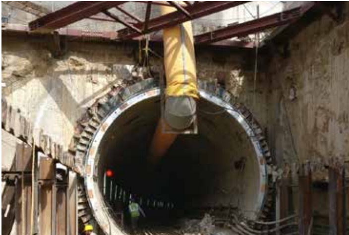
East Bound Tunnel- Launching Shaft Underground Ground-1 From Apparel Park Depot towards Kankaria East
