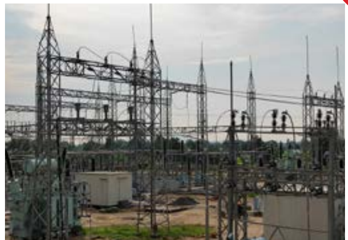
Govindpalli Sub Station-2 under Odisha Transmission System Improvement Project.
