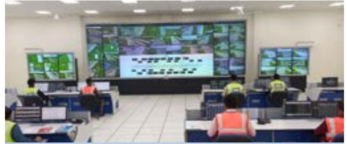
Delhi Eastern Peripheral Expressway (EPE) Intelligent Transport System (ITS) Control Centre.
