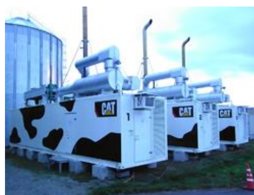
Figure 48 Gas Power Generators
