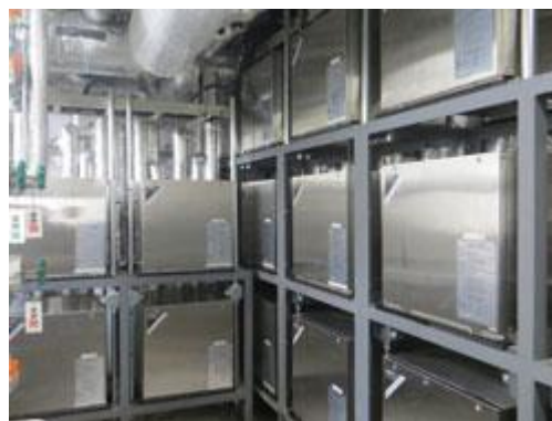
Figure 31 Heat Exchangers in the Community Center
