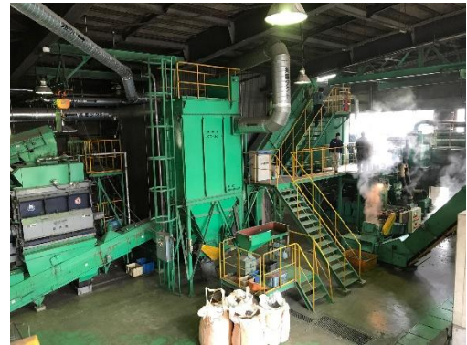
Figure 53 RDF Production Plant
