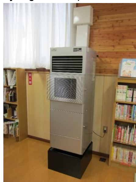
Figure 51 Pellet Stove at Atsuta Elementary School
