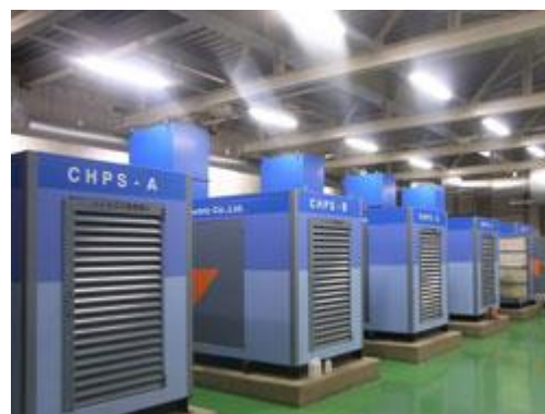
Figure 35 Biogas Power Generators
