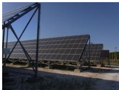
Figure 29 Wakkanai Mega Solar Power Plant
