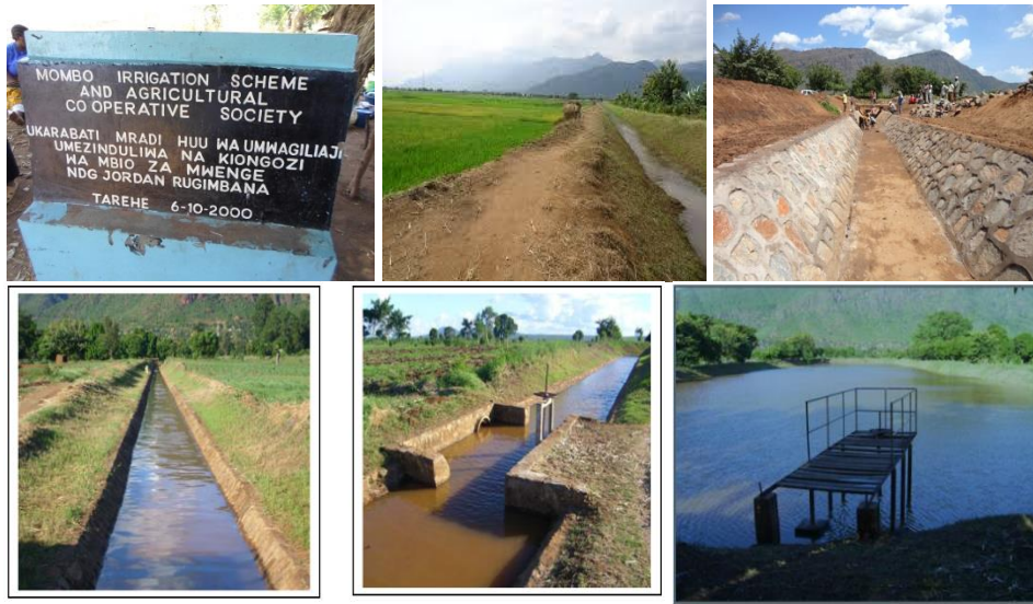
Improved irrigation canals, water gates, night reservoir
