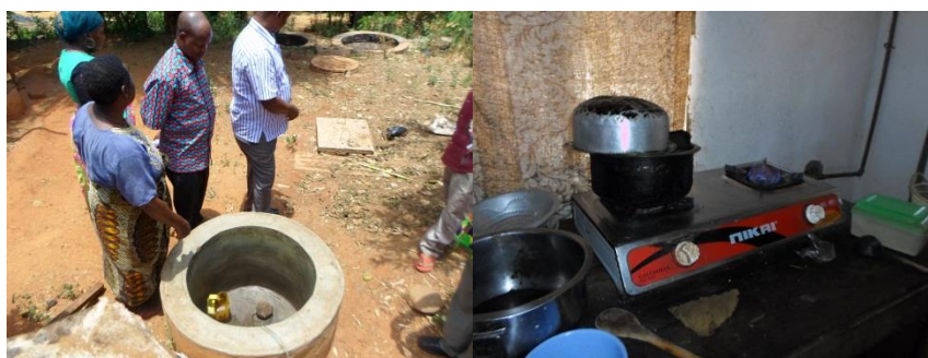
Biogas plant and kitchen equipped with biogas stove
