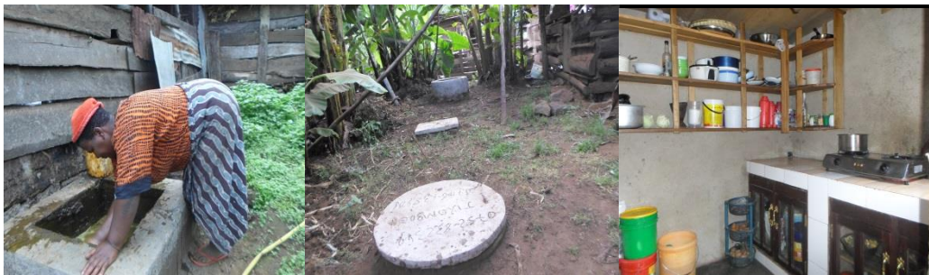
Dairy shade linked to biogas plant that supply energy to the kitchen
