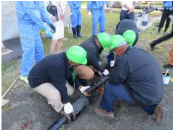
Figure 18 Artificial Leak Occurrence by pressurized Water and Plumbing at Takano Water Treatment Plan, Mie Prefecture
