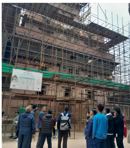
Students observe the ongoing reconstruction works at the Degu Taleju Temple in Patan Durbar Square which is supported by the Government of Japan.
