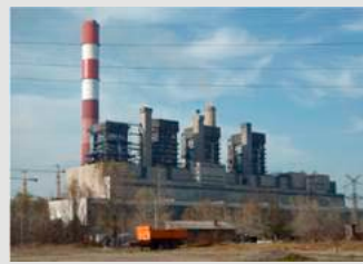
Flue Gas Desulphurization Construction Project for the Thermal Power Plant Nikola Tesla
