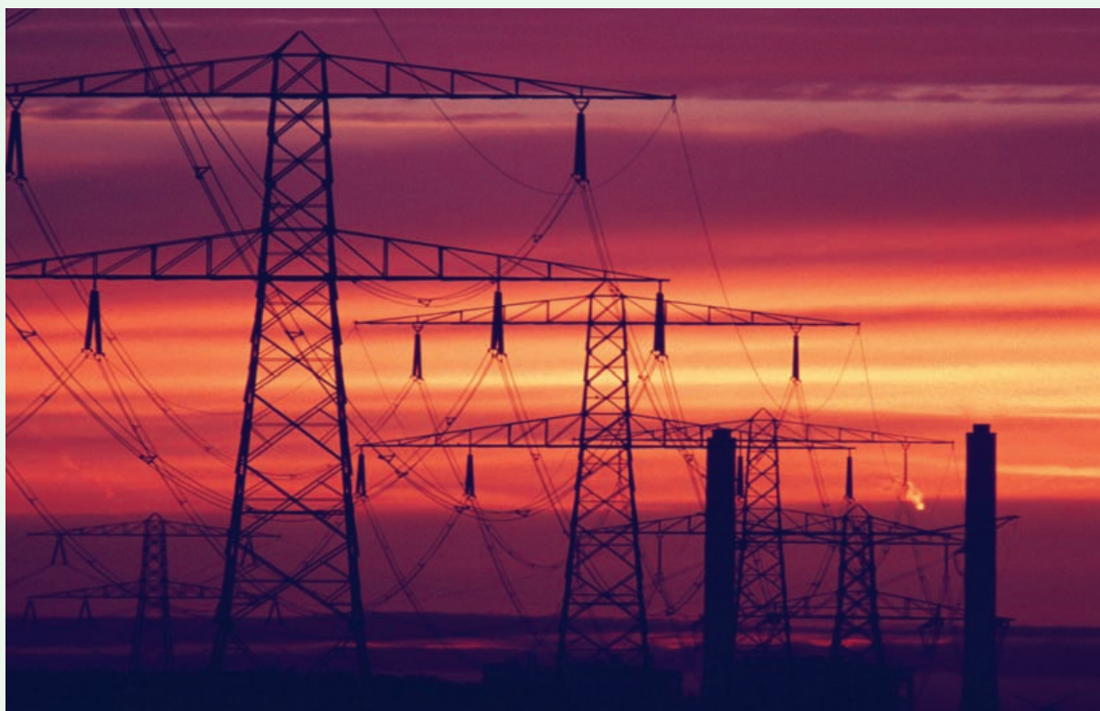
Growing power lines reflect dynamic infrastructure development
