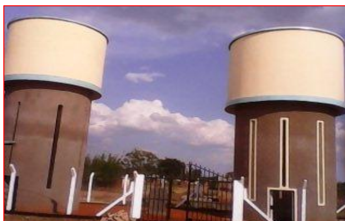
Left the 45,000lts tank and right is the 90,000lts capacity
