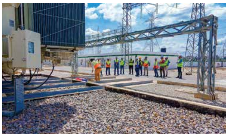
Zuzu Substation in Dodoma [Photo: TANESCO]
