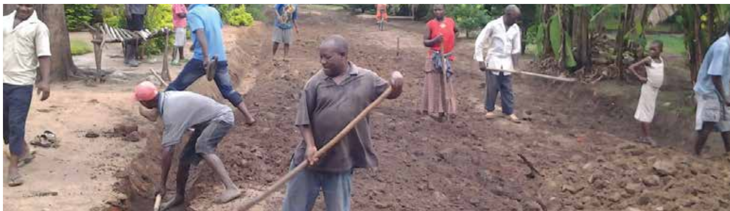
Villagers in Mang'ula B constructing Community Road by using O&OD methodology, which is “Self-Help Efforts” of the communities to deepen collaborative relationship between Local Government and Communities.
