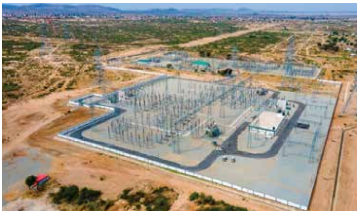
Aerial photo of Zuzu Substation in Dodoma (Photo: TANESCO)
