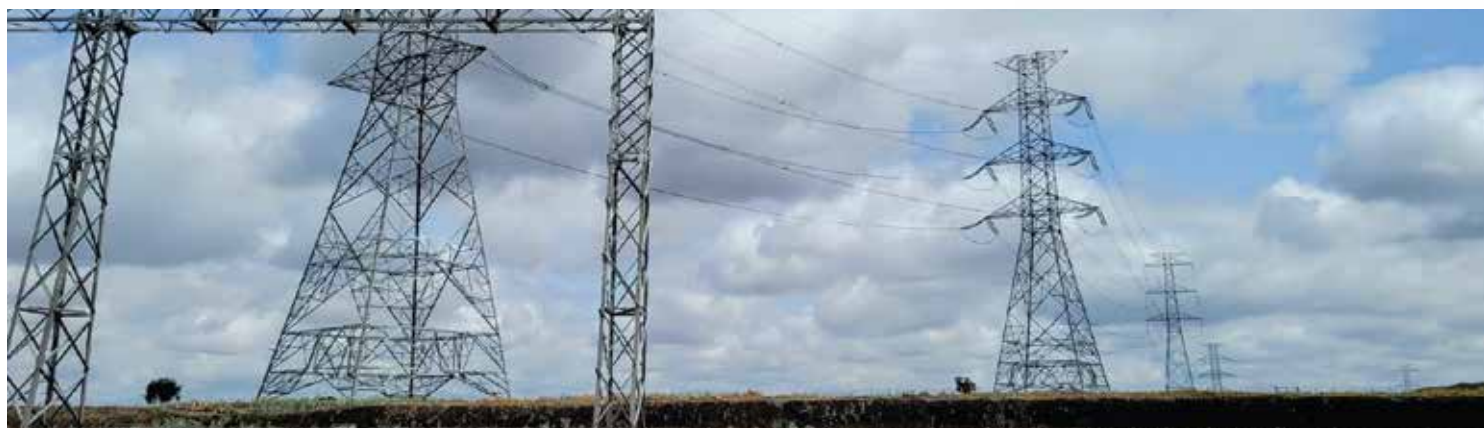
400KV transmission lines
