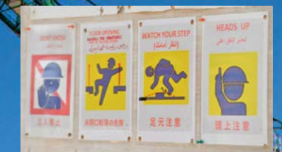
A total of about 25 Japanese and Palestinians are working together at the construction site. At the site precautionary measures are taken place, such as displaying warning signs just like in Japan. Sharing and introducing the culture of safety is also an important part of the mission.
