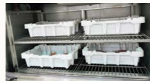
Above: Storing seafood in Kubaran, the high-level refrigeration equipment.
