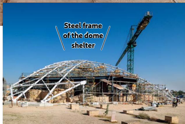
The shelter area is 55 x 45 meters, and its height is about 13 meters.
