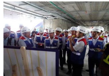
Pham Binh Minh, the deputy prime minister of Vietnam inspection at the urban railway construction site
