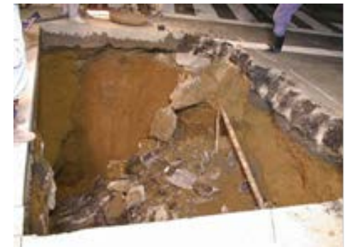
Major road collapse
