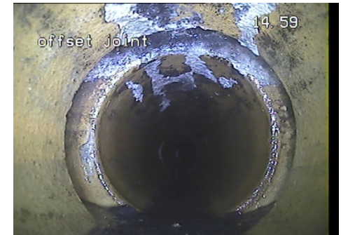
Open joint due to poor installation
