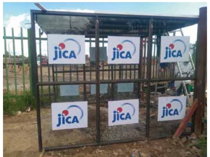
Full Body Sanitizer installed at Kasumbalesa Walkway
