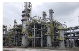
Natural gas production plant in Pertamina
