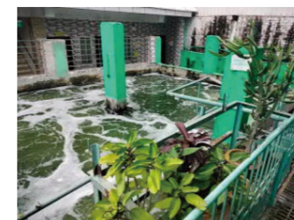
Wastewater treatment plant for a facility for cleaning garments for export, which was built with a loan from the Bangladesh Financial Sector Project for the Development of SMEs
