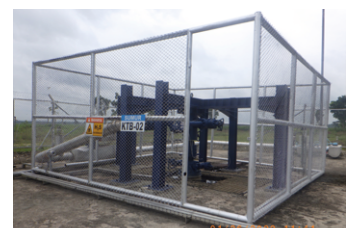
A well planned for CO 2 injection in the Gundih gas field
