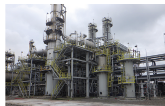
Natural gas production plant in Pertamina
