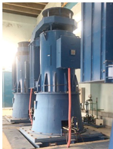
Drainage Pumps Installed under the Project
