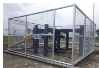
A well planned for CO 2 injection in the Gundih gas field
