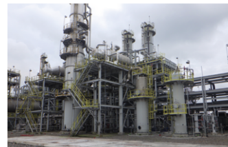
Natural gas production plant in Pertamina
