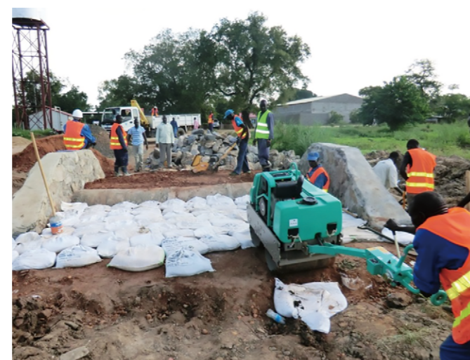
On-the-job training on repairs using sandbags for The Project for Capacity Development on Sustainable Road Maintenance and Management in Juba, South Sudan (September 2013)
