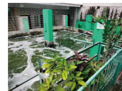
Wastewater treatment plant for a facility for cleaning garments for export, which was built with a loan from the Bangladesh Financial Sector Project for the Development of SMEs
