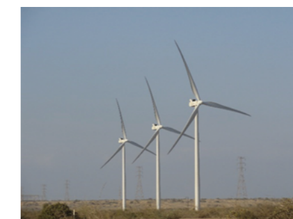
Wind power plant financed by the Peru Energy Renovation Infrastructure Assistance Program
