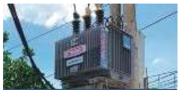
Amorphous transformers in power distribution, Yuko-Keiso, Vietnam
