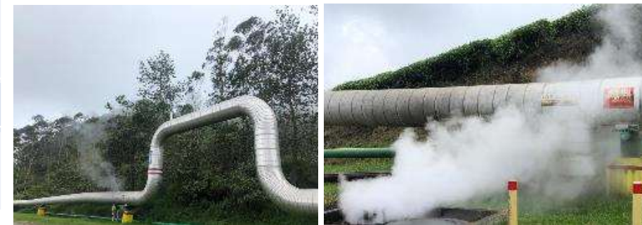
Geothermal steam pipes
