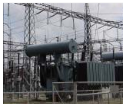
Figure-5: 300 MVA Transformer
