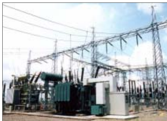
The Concepcion substation
