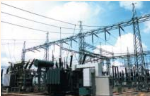
The Concepcion substation
