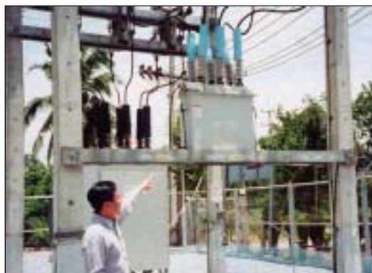
Site Photo: Ang Thong 1 Substation
