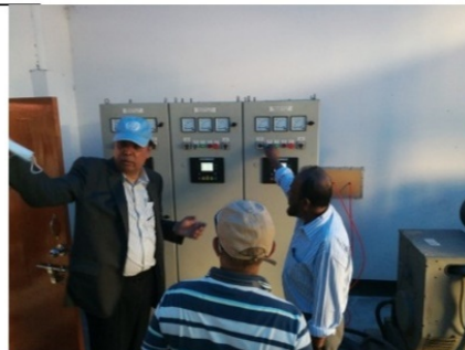
Control room of biogas generator
