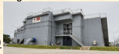
U-BCF installed in Hai Phong, Vietnam
