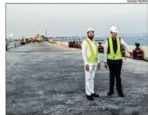
CM Eknath Shinde and Dy CM Devendra Fadnavis on the Mumbai Trans Harbour Link, the deck work of which was completed on Wednesday
