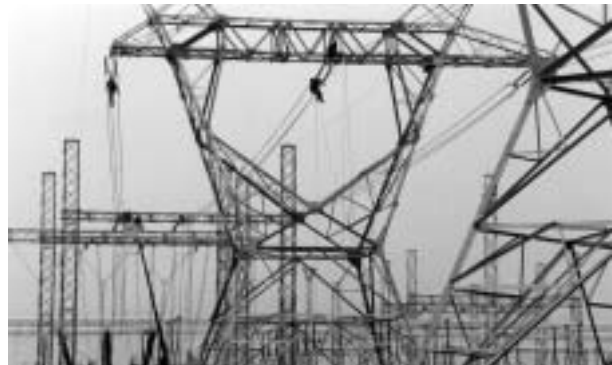
Transmission lines financed by untied loan
