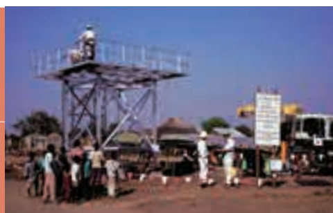
Construction site of a water supply facility: Development of basic infrastructure is urgently required in Sudan. (Emergency Study on the Planning and Support for Basic Physical and Social Infrastructure in Juba Town and the Surrounding Areas)
