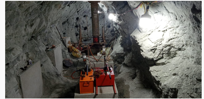
Draft Tunnel Investigation at the Project for the Construction of Turga Pumped Storage (I)
