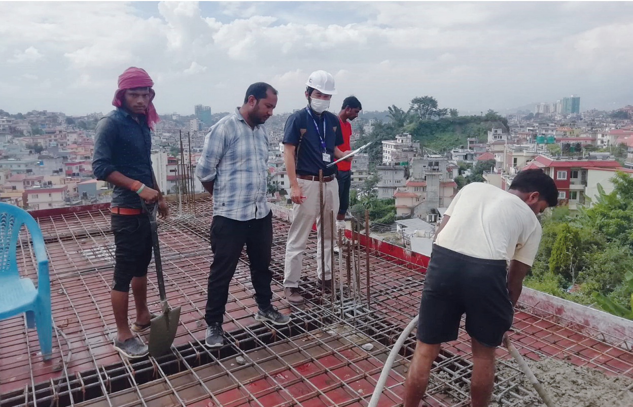
Conducting a baseline Survey on building code compliance at a construction site
