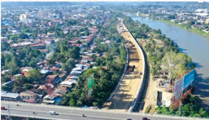
Flood Risk Management Project for Cagayan de Oro River, photo courtesy of Toyo Construction Co. Ltd.
