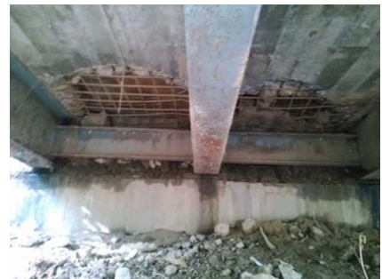
Disintegration of RC deck (This damage is caused by over loaded vehicles.)
