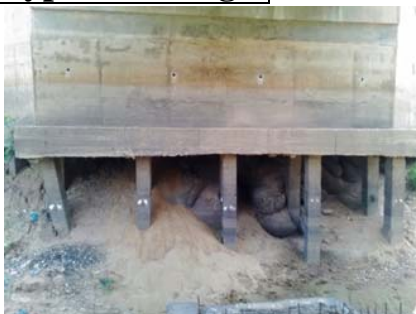
Scouring around and under abutment (Soil under abutment was lost and exposes all pile)
