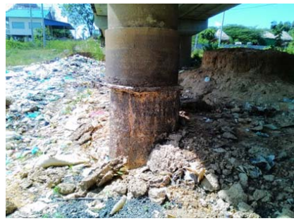
Scaling and exposing rebar on surface of column by scouring
