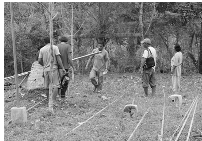
COFFEE NURSERY. Sulu coffee farmers (above photo) are shown setting up the construction materials of the coffee nursery farm site after laying out this site at Kandayok, Panamao, Sulu island.
