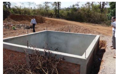
Special pit for the disposal of healthcare waste under construction in XYB
