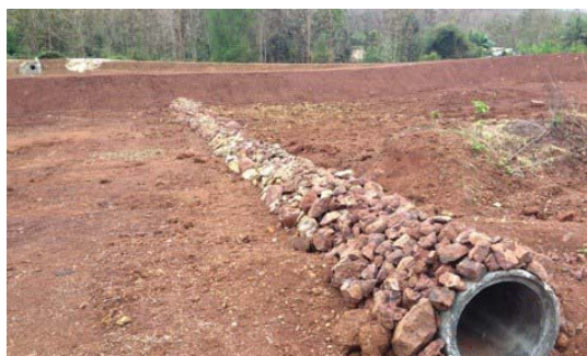
Leachate collection pipe installed at KM8 in Luang Prabang. Leachate is highly polluted water that generates from waste dumps. This will be the first-ever leachate treatment system in Laos.
