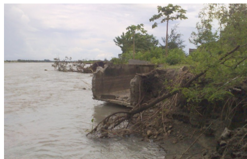
Approximately 900 meters of the main canal connected to the main intake was washed out as water overflowed from Bucao River. PHP 15 million is needed for its repair and restoration.
