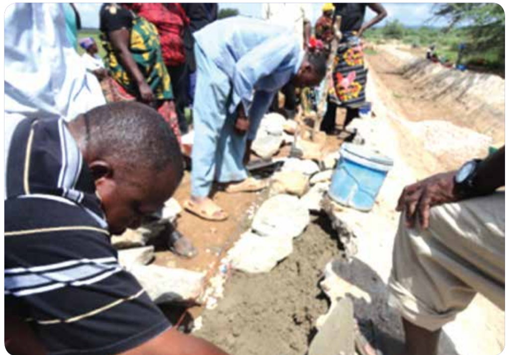
Participatory repair work of irrigation canal. IO members implemented capping technically supported by district and zone staff.
