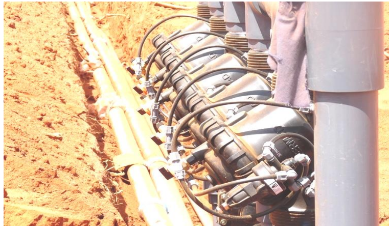
Drip irrigation Pumps and Underground Pipes
