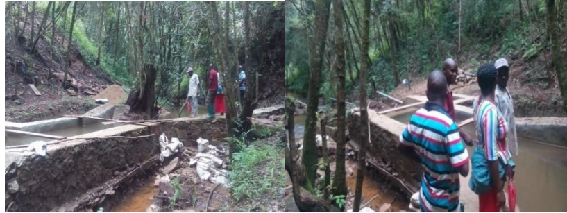
Water intake at Igongwi Mountain ranges
