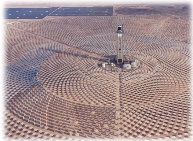
A solar thermal power plant in the Atacama Desert
