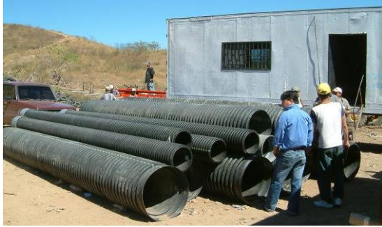
Photo 7-16 Leachate Collection Pipes
