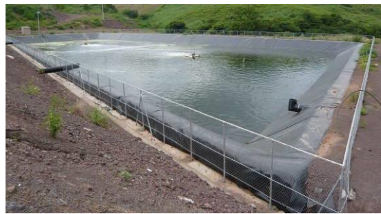
Photo 7-19 The Use of Aerators in the Leachate Pond
