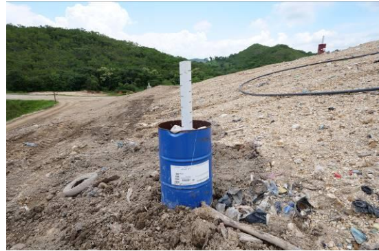
Photo 7-39 Gas Venting Pipes
