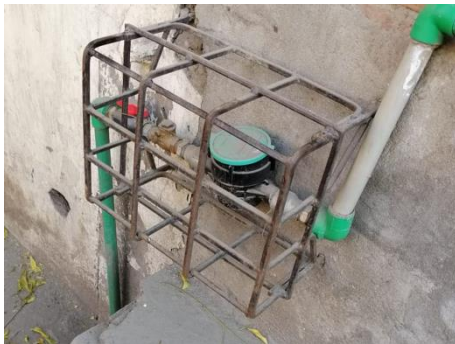
Situation of meter installation
