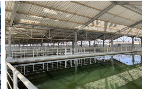
Water purification area
