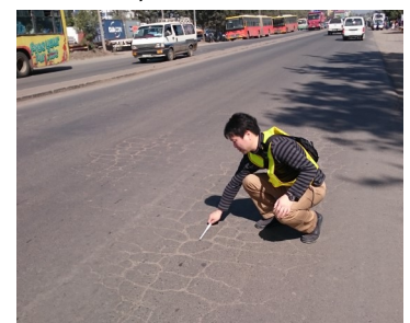
Japanese expert measuring road damage.
