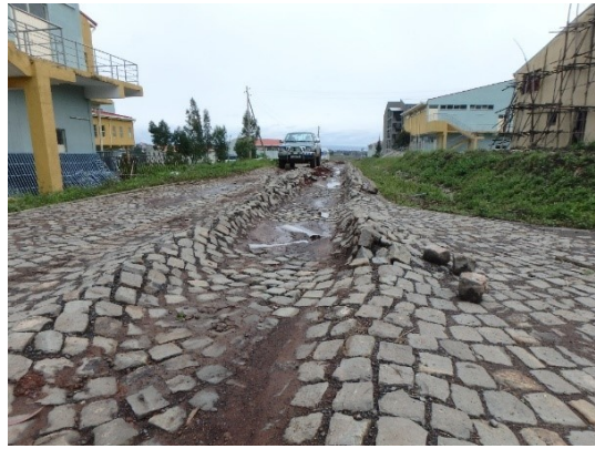
Distorted roads due to expansive soil
