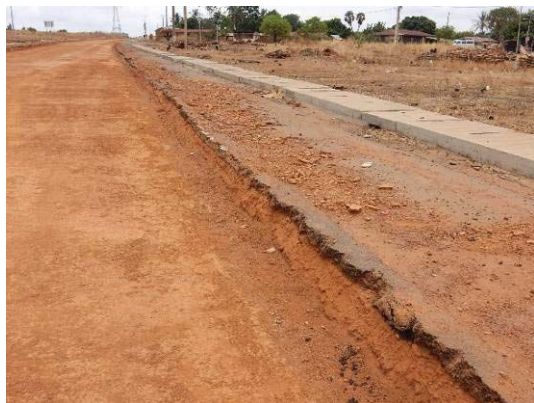
After Removal of Cement stabilized Base Course on Bafilo Bypass in Togo
