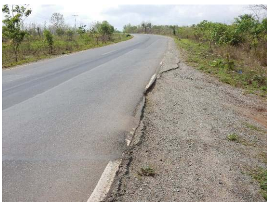
Edge damage on central corridor in Togo
