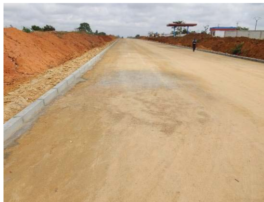
Completion of Cement Stabilized Sub-base Course on Lomé - Tsevie Section in Togo
