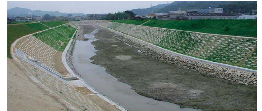
Reconstruction of the embankments of the Sumoto River that suffered damage from a downpour caused by typhoon No. 23 in 2004 (Sumoto City)
